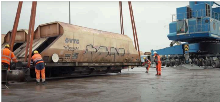
The decommissioned wagons are carefully lifted from their sidings and into Thompson's Decom facility at the Port of Blyth.
